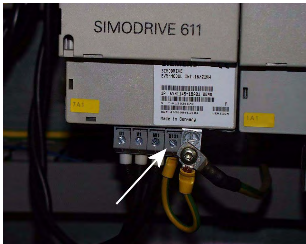
Photo: Siemens E/R module with terminal X131
