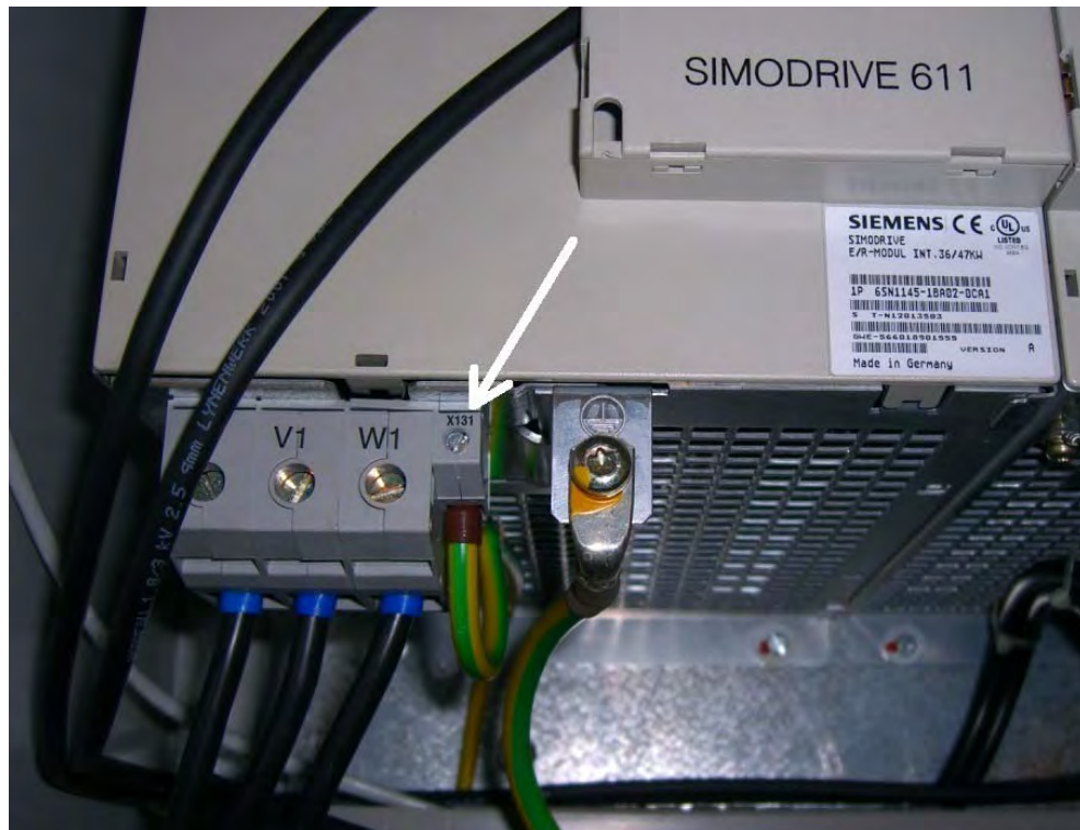
Photo: Siemens E/R module with terminal X131
