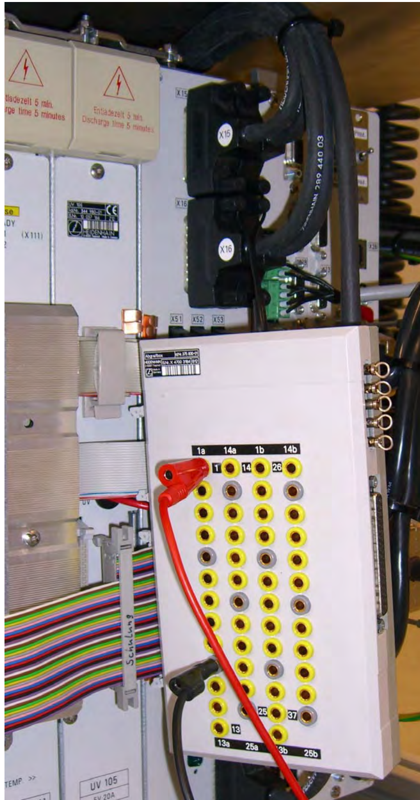
Photo: Connection of the test adapter to the power supply bus
