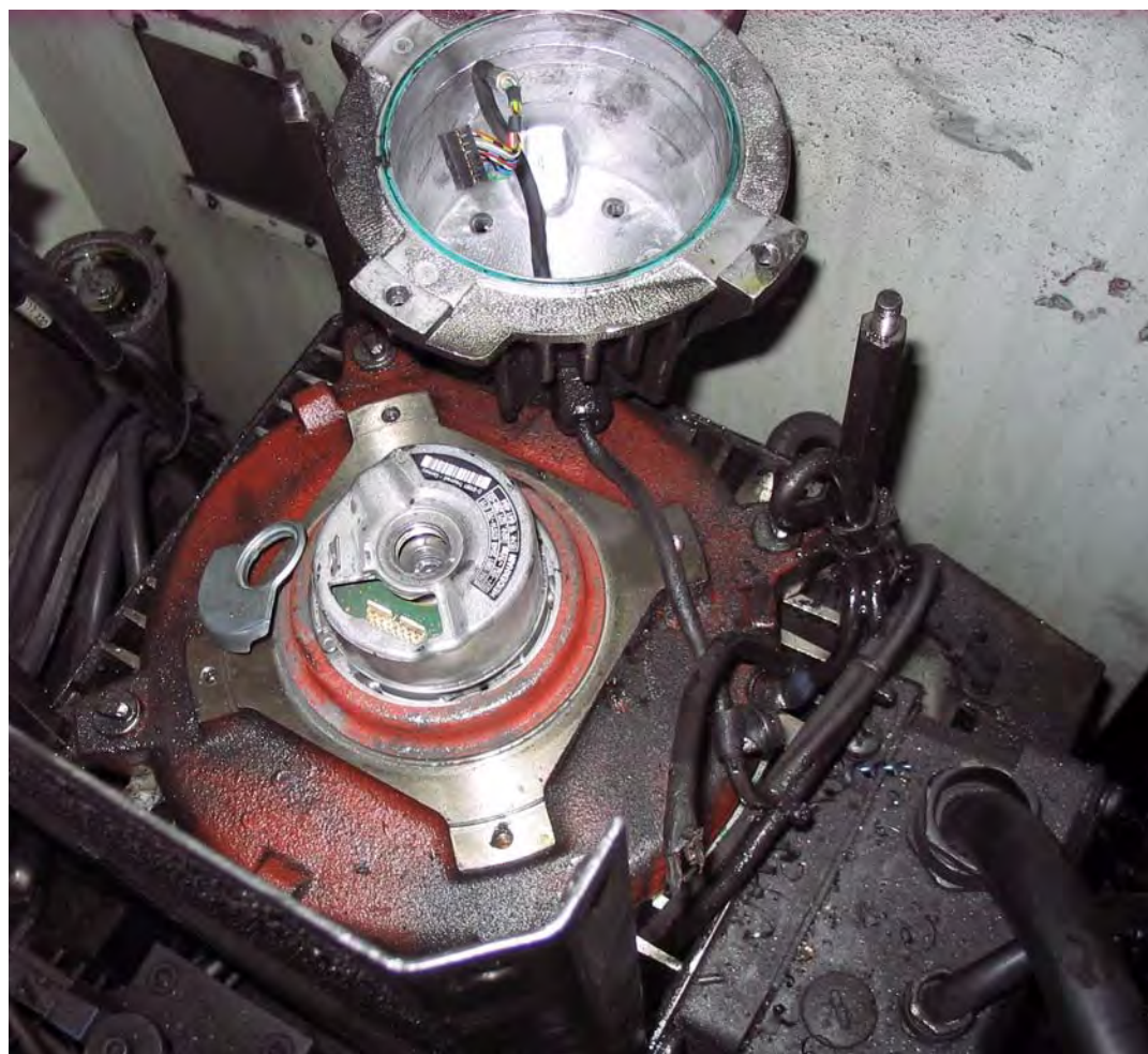
Photo: Defective and heavily contaminated motor
