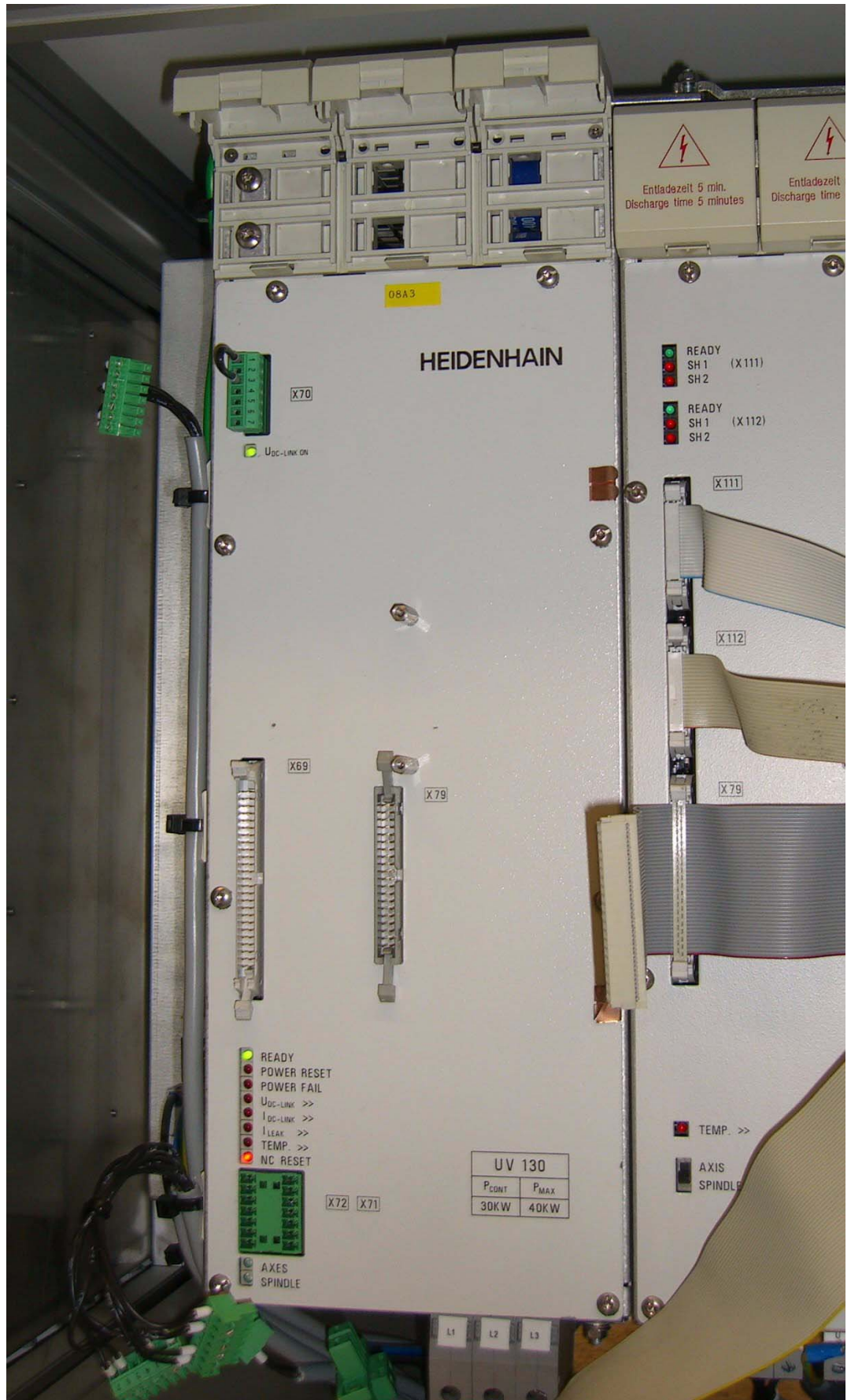
Figure: UV without connected units
