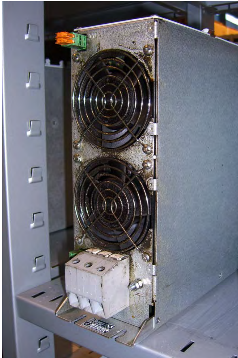
Photo: Heavily contaminated inverter
