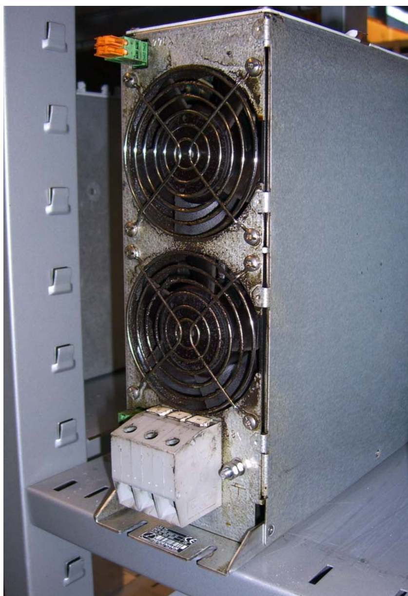
Phot: Severely contaminated inverter
