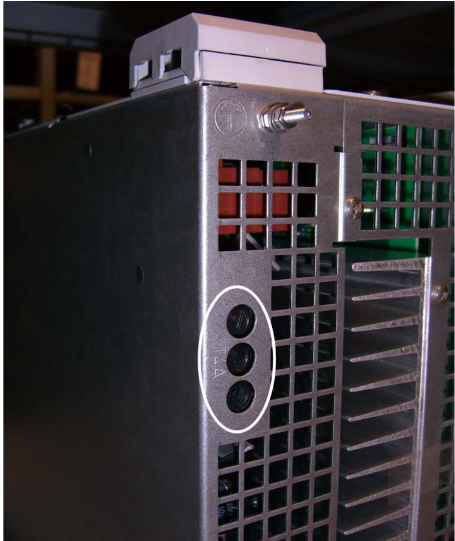
Photo: Location of the fuses
