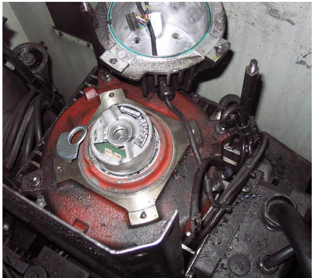
Photo: Defective and severely contaminated motor
