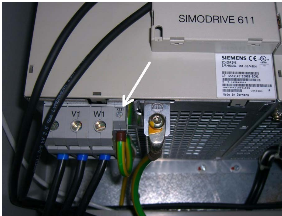
Photo: Siemens E/R module with terminal X131
